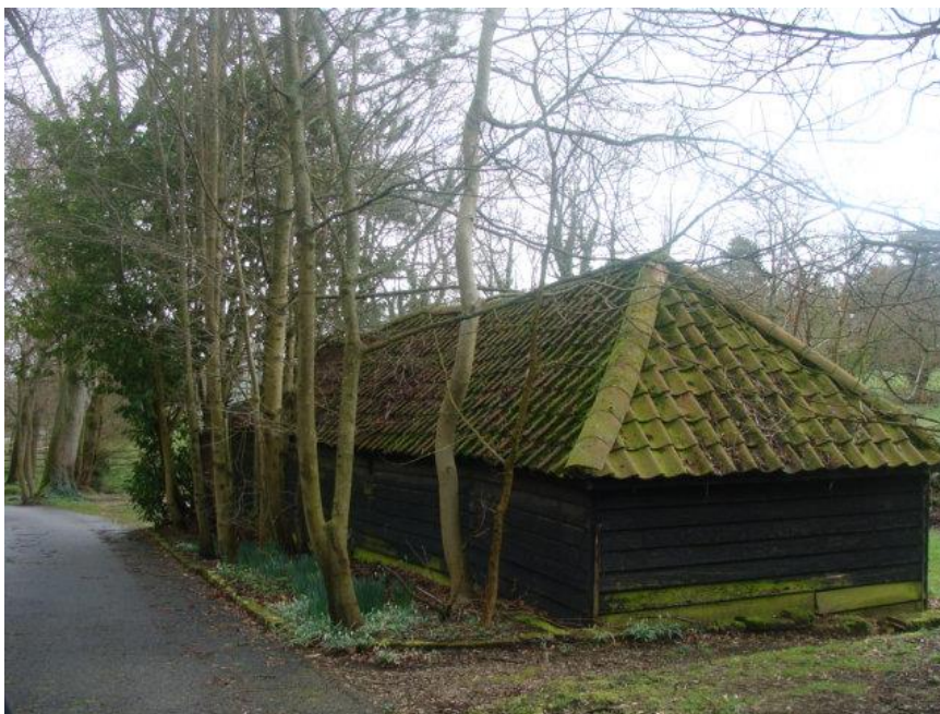
Picture 22. Simple barn dating from late 19th/early 20th century most worthy of retention.
